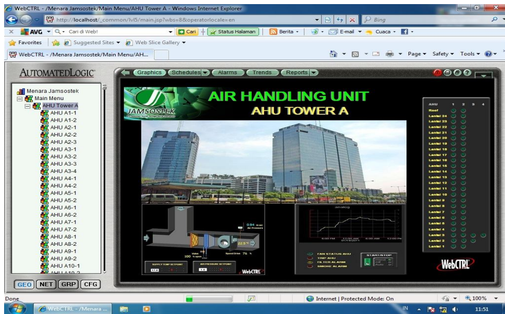
Gambar 14. Tampilan AHU Tower A
